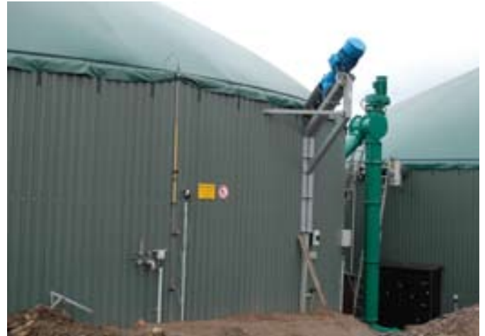
Neue Biogasanlage in Ober-Seemen
